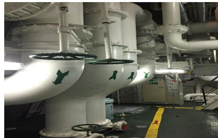
BWTS Piping in Engine Room
