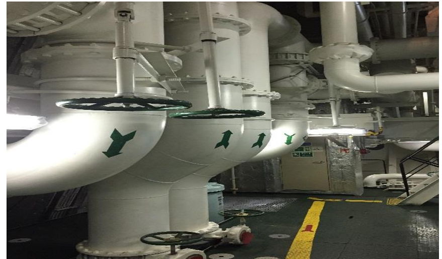
BWTS Piping in Engine Room
