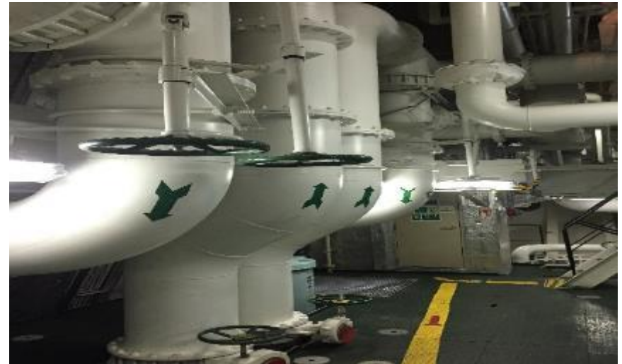
BWTS Piping in Engine Room
